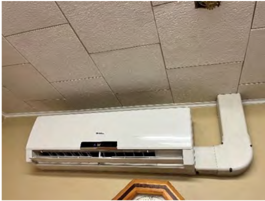
Figure 12 Indoor Unit in Office Area
