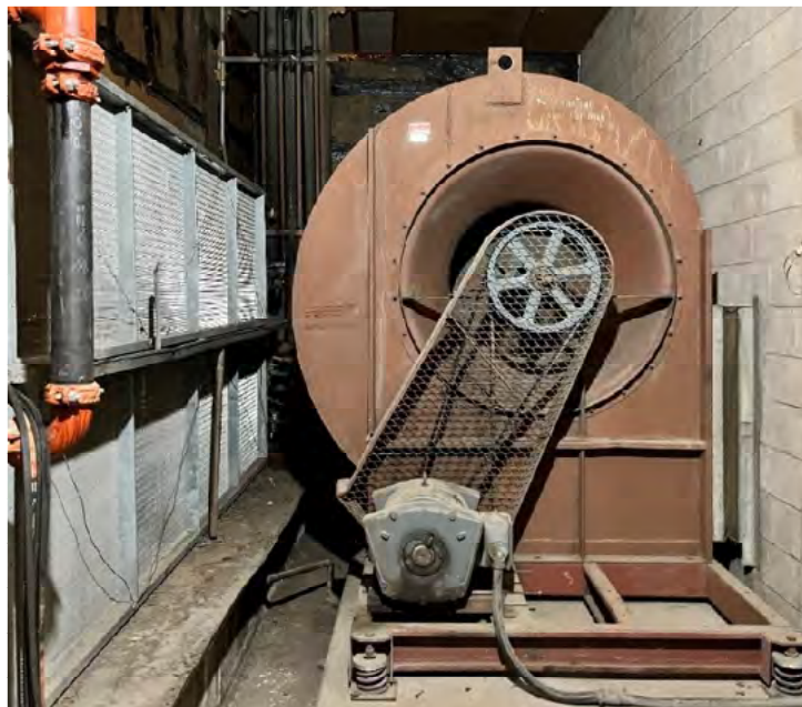
Figure 6 Built-up Air Handling Unit
