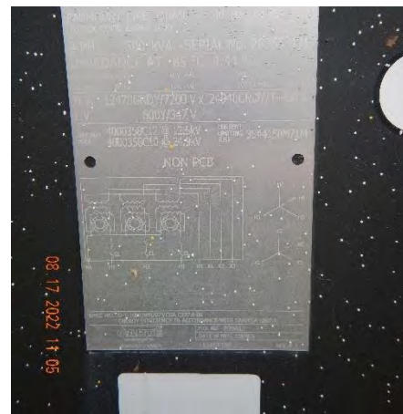
Figure 2: Utility Transformer Tag
