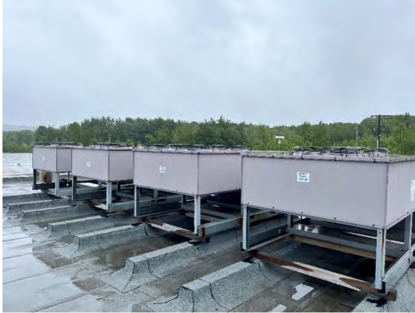
Figure 7 Condensing Units on Roof
