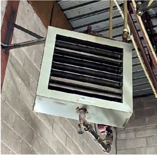
Figure 9 Unit Heater Connection
