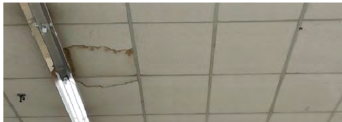
Figure 22 Ceiling water damage in retail space from leaking Victaulic joints
