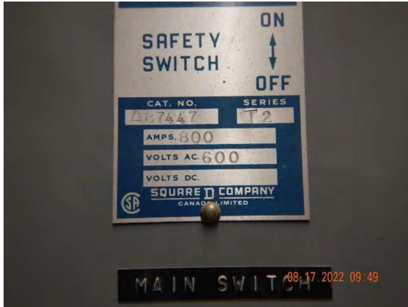
Figure 3: Main Disconnect Switch
