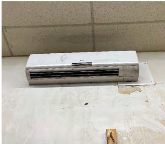
Figure 14 Indoor Unit in Storage Area
