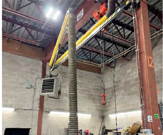
Figure 10 Unit Heater in back of Facility
