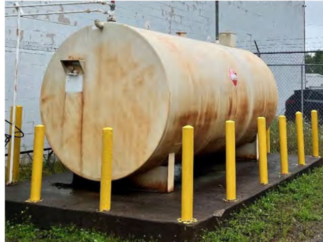
Figure 5 Fuel Oil Storage Tank
