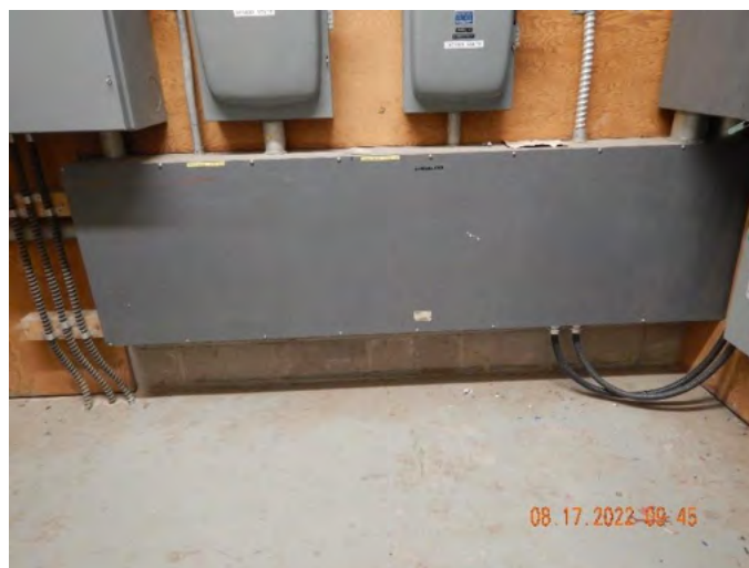
Figure 4: Main Building Splitter
