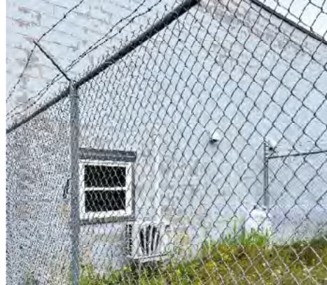
Figure 13 Outdoor Unit of Office Area
