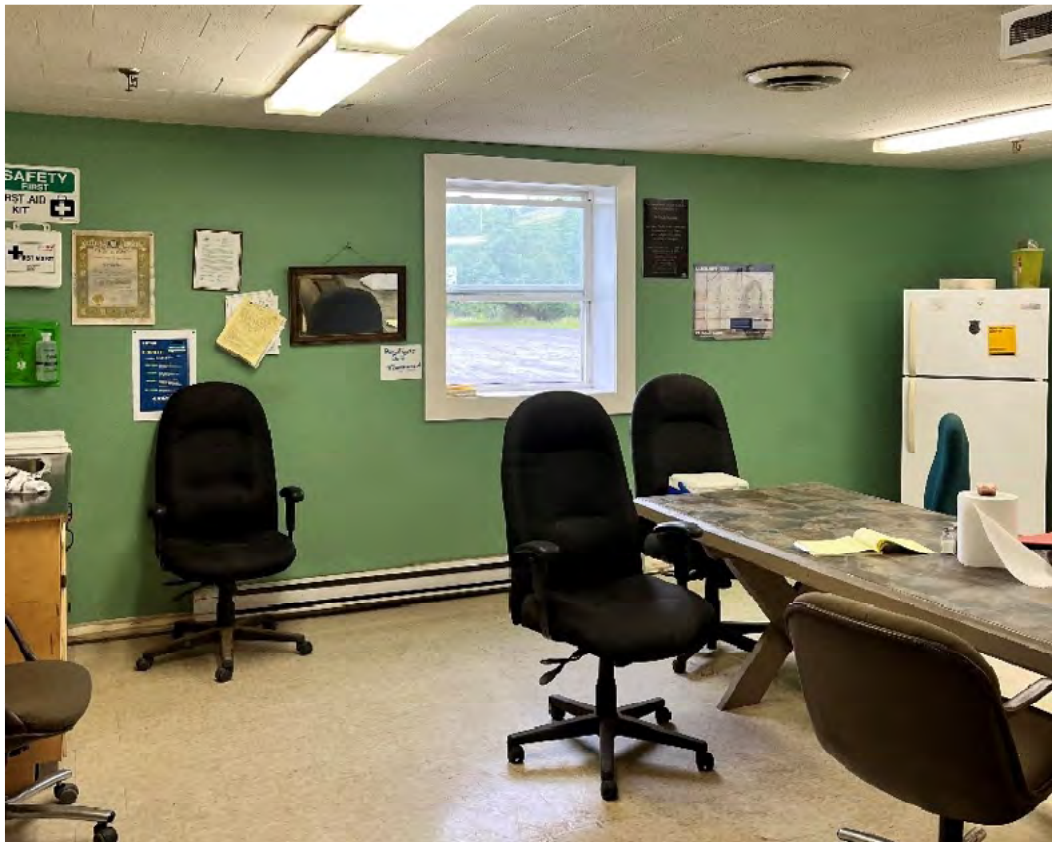
Figure 11 Electric Baseboard in Breakroom
